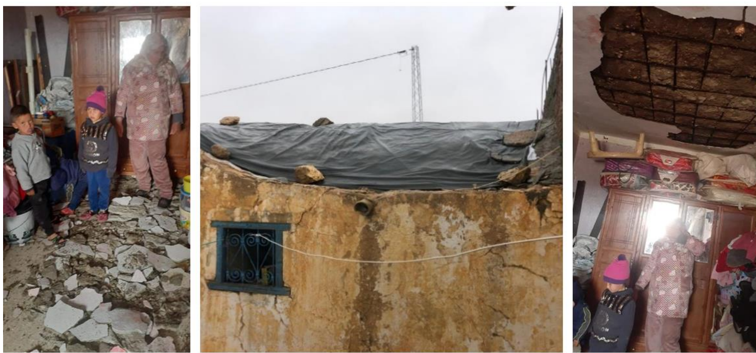
Figure 5: Losses and damages caused by flash floods. Credit: TRC
