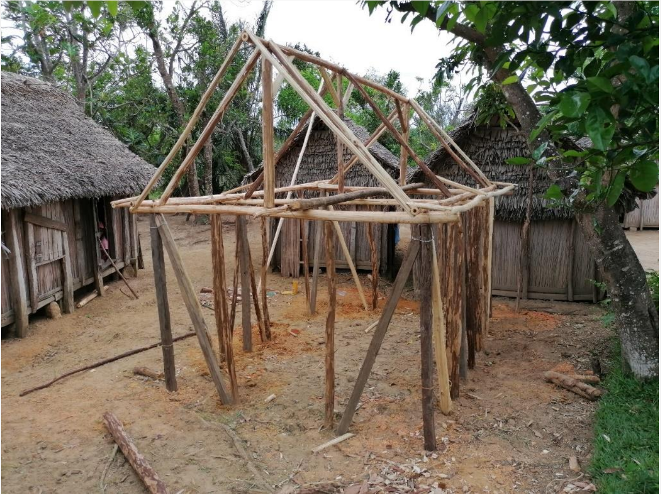
A shelter reinforced with bracings under construction in Sandrohy (Photo credit: Pascal Panoseti, IFRC)
