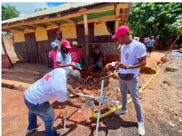
The Spanish Red Cross is supporting the HRCS to provide SETA units for water treatment and distribution. Source: Spanish Red Cross.
