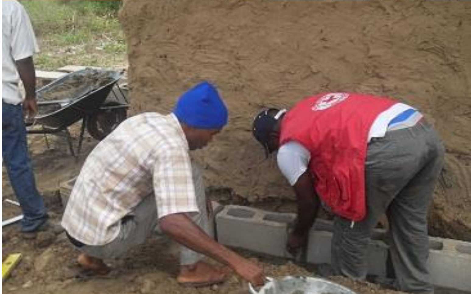
Early recovery shelter construction in progress in Ozahi (i) and Odogwu (ii)
