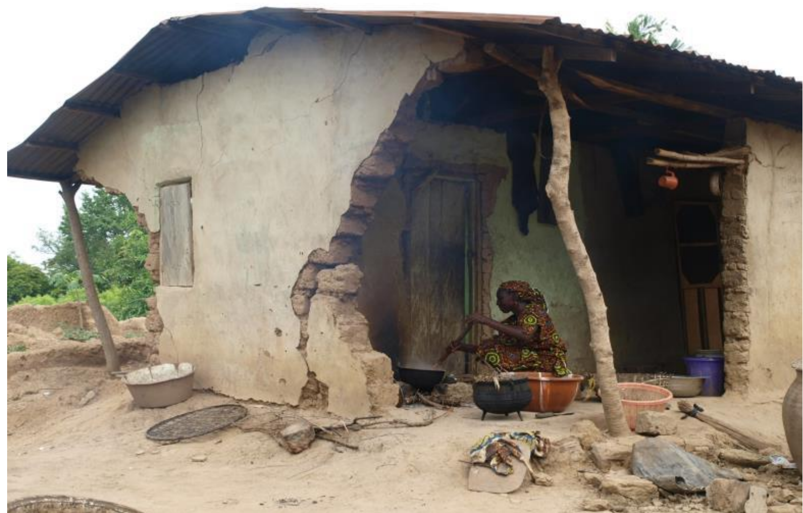
Flood damage caused to people's homes in Mozum Ose and Ozahi
