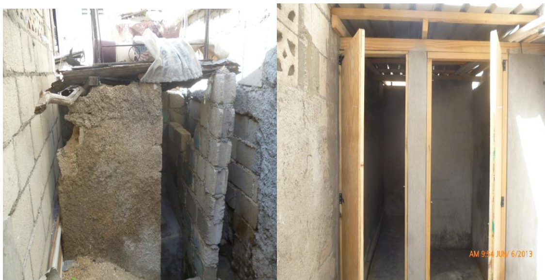
One of the repaired toilets (before and after the intervention). Source: IFRC
