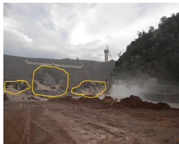
Water seen gushing through the collapsed parts of the dam wall marked in yellow. Photo ZRCS 06.02.14
