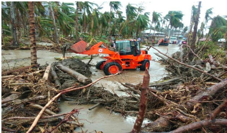
Continuous clearing operations activity by PRC-Southern Leyte in Municipality of Libagon, Southern Leyte (Photo: PRC)
