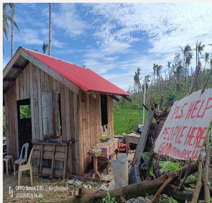
Three (3) days after distribution, some houses in Siargao started repairing their roofs (Photo:PRC)
