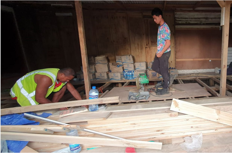
Significant warehouse repairs at TRCS national headquarters have been completed to prevent damage to relief items. Photo: TRCS
