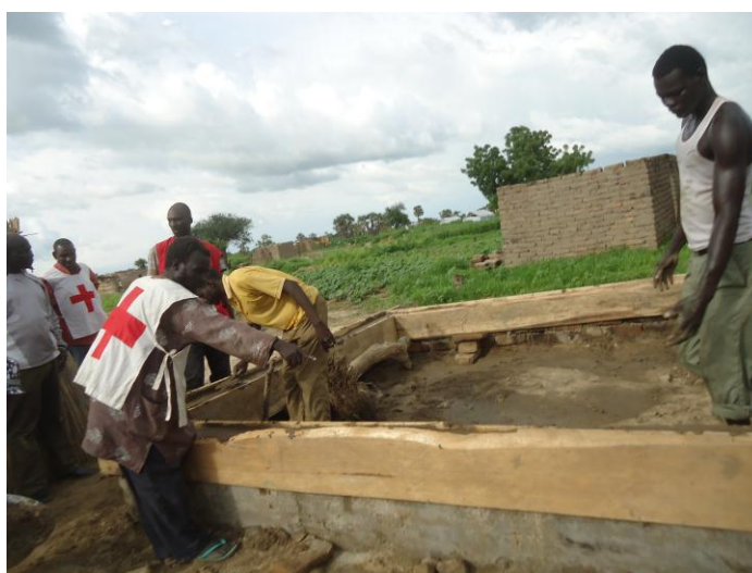
Construction of solid foundations by CRC volunteers in the locality of Blangoua, Far North Region of Cameroon Source: Cameroon Red Cross
