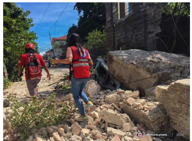
Several houses and infrastructures in different locations were severely damaged after the 7.0 magnitude earthquake in Tayum, Abra. PRC volunteers were mobilized to provide assistance (Photo: PRC).
