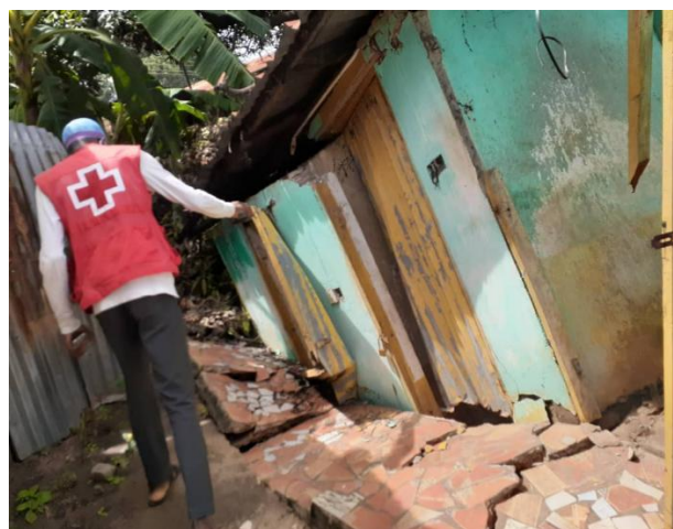
A partially collapsed building. Photo by GRCS
