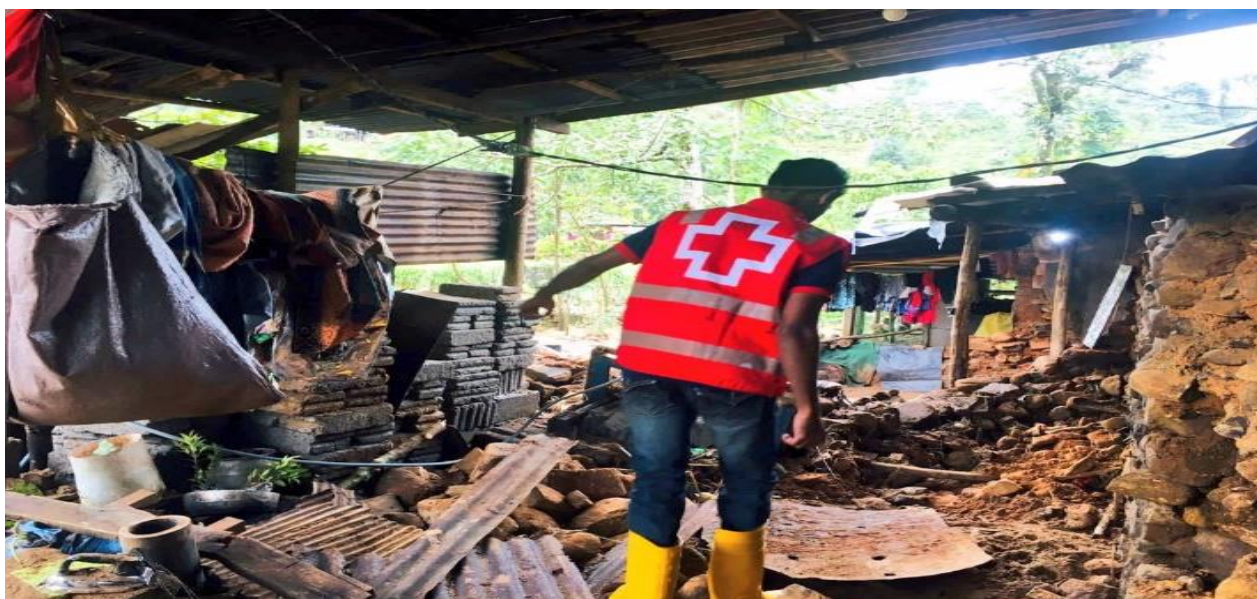
SLRCS BDRT members inspecting the damages to houses (Photo: SLRCS)
