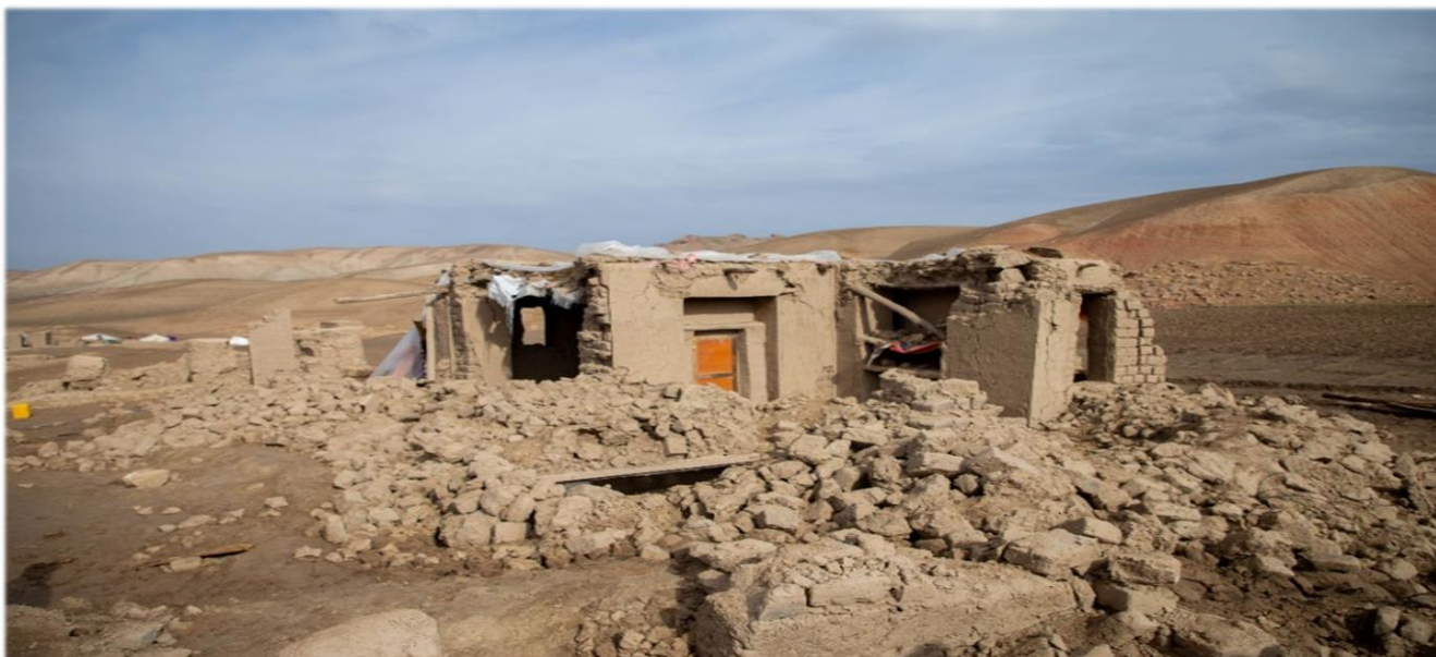
A house destroyed by the earthquake in Qadis district of Badghis province, January 2022. (Photo: Meer Abdullah/IFRC)
