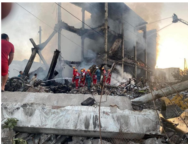
Assessment and search and rescue operation by ARCS' volunteers around the three-floor building that was destroyed by the explosion
