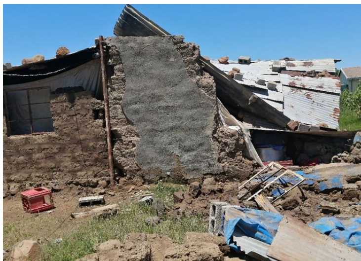
Figure 1: Partially destroyed house in OR Tambo District
