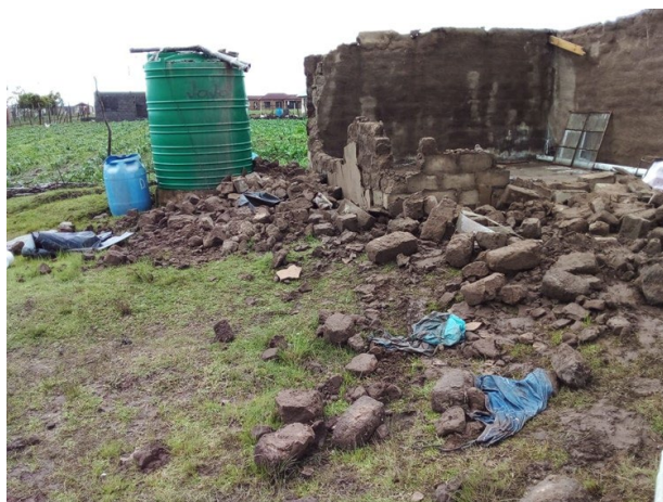
Figure 3: A destroyed house in Buffalo City District
