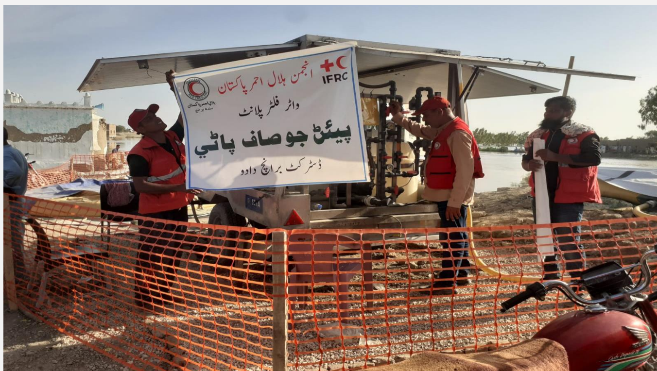
A water treatment plant being installed by trained PRCS staff in Dadu, Sindh. (Photo: PRCS)
