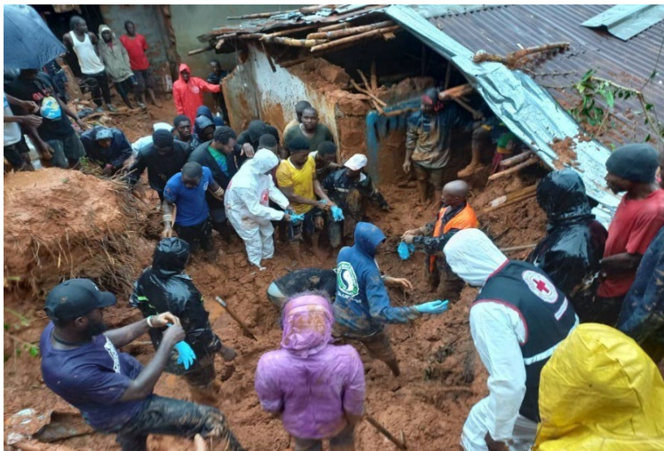
SLRCS Volunteers supporting rescue in a collapsed building (Photo: SLRCS)
