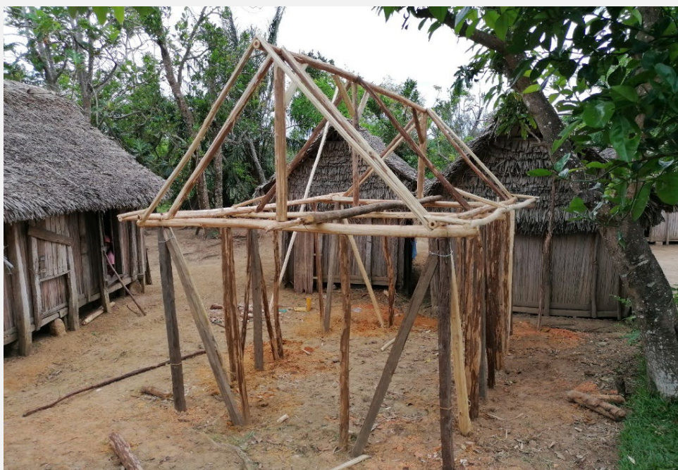
Figure 3: A shelter reinforced with bracings under construction in Sandrohy (Photo credit: Pascal Panoseti, IFRC)
