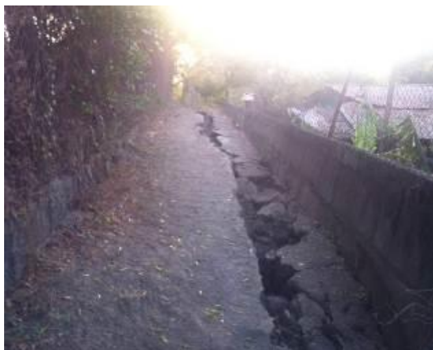
Activation of geological faults in communities Matiare municipality, department of Managua, Nicaragua. Source: IFRC.
