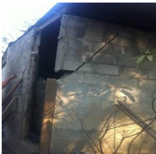
Housing affected by the earthquake in the municipality of Matiare; is observed the use of wood as a combined column with a wall of blocks. Source : IFRC.
