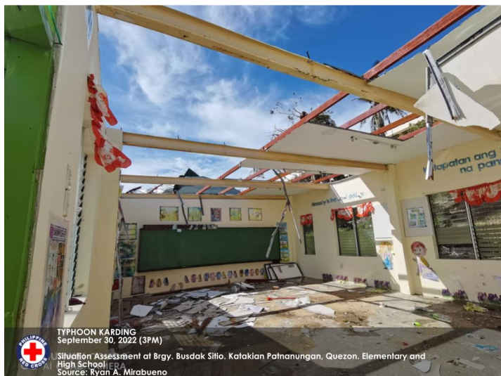
Damaged school in Quezon (Source: Ryan A. Mirabueno)
