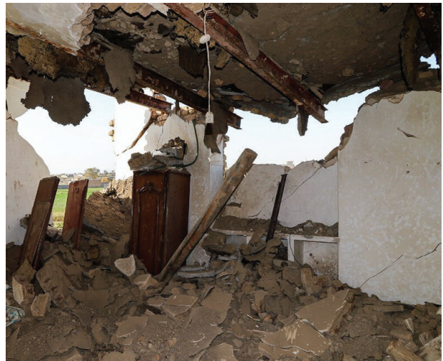
Building damages caused by the earthquake. Credit: IRCS
