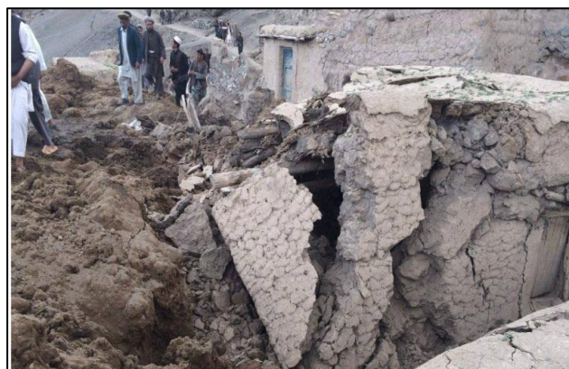
Damage caused by the twin landslides in Abi Barik village, Argo district, Bhadhakshan province. Photos: IFRC.
