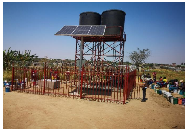
Picture showing the whole Piped Water Scheme Structure at Hopley Borehole 1 as beneficiaries access water.
