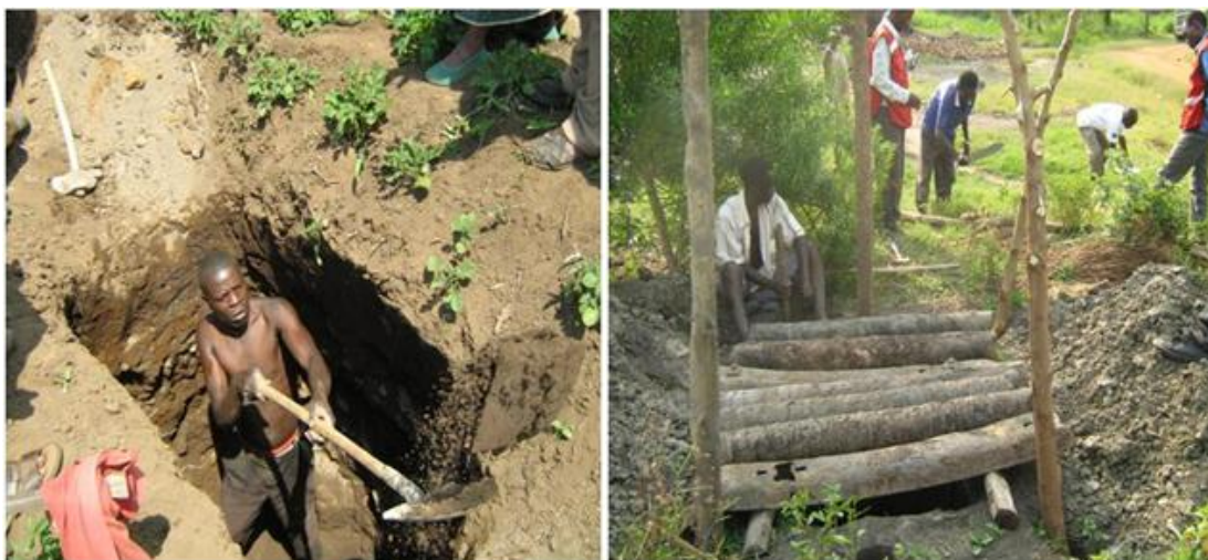
Mobilised locals engaging in the sinking of latrine pits, Red Cross volunteers following up use of tools and latrine construction sites Photo: URCS.
