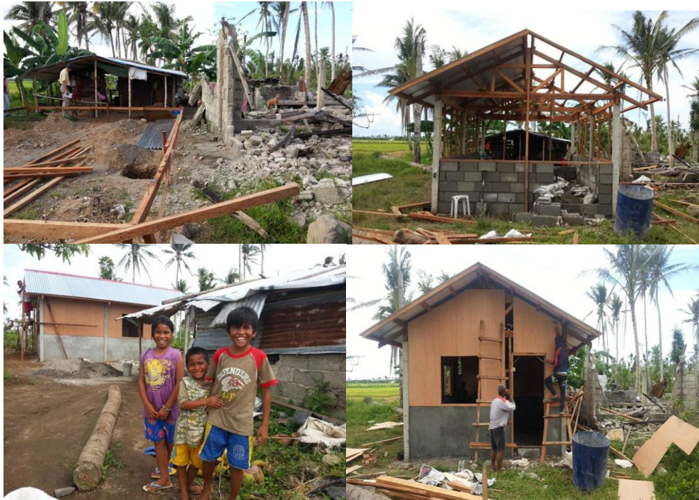
(Clockwise from the top left) The building of core shelter housing in Tabontabon began in April and now continues, expanding across several municipalities in Leyte. Consisting of both timber and concrete, these shelters will provide more resilient housing for families in the upcoming storm season this year. (Photo: Jonathan Brigham/IFRC)
