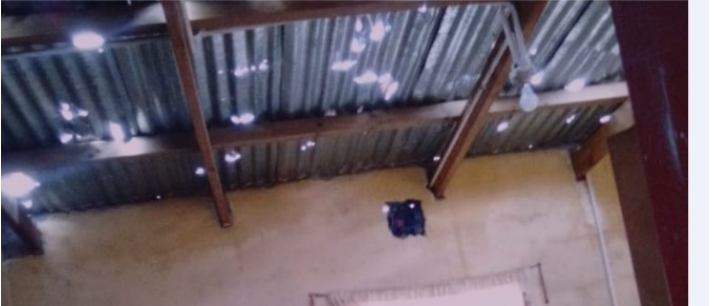
Roof destroyed by hailstones, as assessed by BERCS
