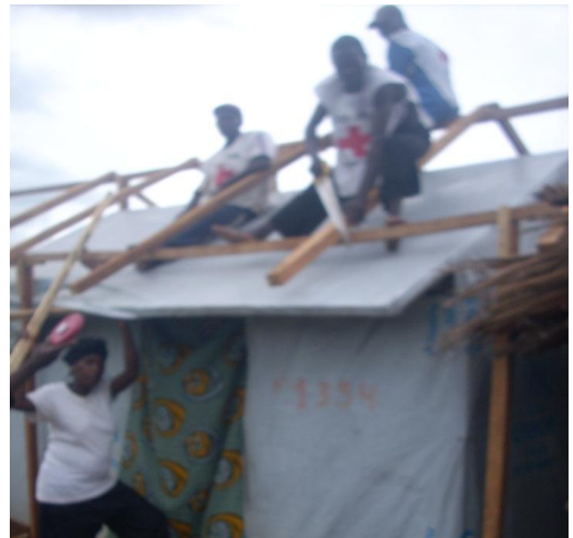
Semi-permanent shelters under construction by DRC Red Cross volunteers (Photo: DRC Red cross)
