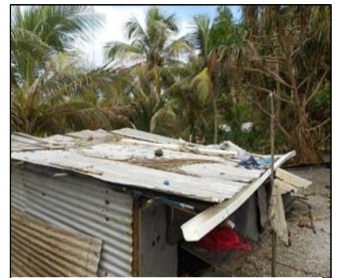
Gutter in need of repair is identified during an IFRC WASH household survey conducted in August 2013 of Majkin Island, Namu Atoll. Credit: Ana Zarkovic/IFRC
