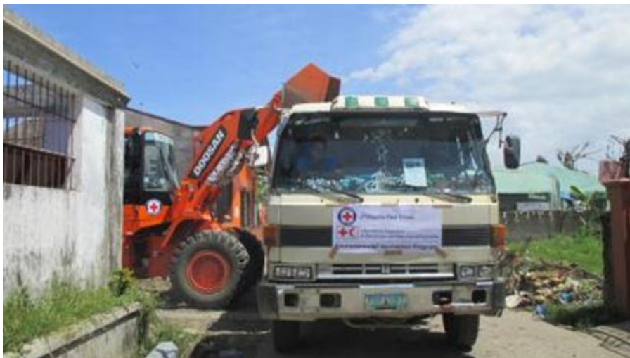
Up to 410 cash-for-work beneficiaries and skilled machine operators helped remove 1,910 m 3 of debris in four municipalities in Leyte. They were supported by PRC staff and volunteers, including registered nurses who helped dispense prophylaxis to workers to prevent any occurrence of leptospirosis. (Photo: PRC/IFRC)
