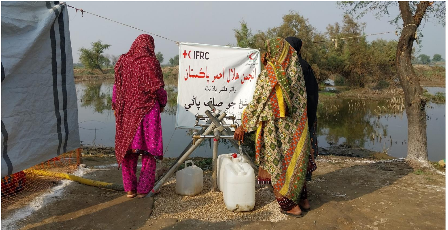
PRCS with the support of IFRC installed a water treatment plant in flood-hit community in Larkana, Sindh to meet the growing need for clean and safe drinking water. (Photo: Angbeen Sohail/IFRC)
