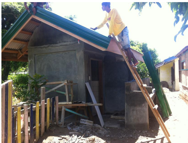
A water and sanitation facility for Abuleg Elementary School, Dinalungan Aurora province constructed through this appeal is being finished.
