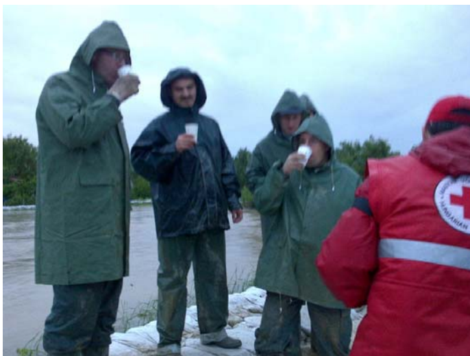
Red Cross support during the flood defense works on the dam. Photo: HRC
