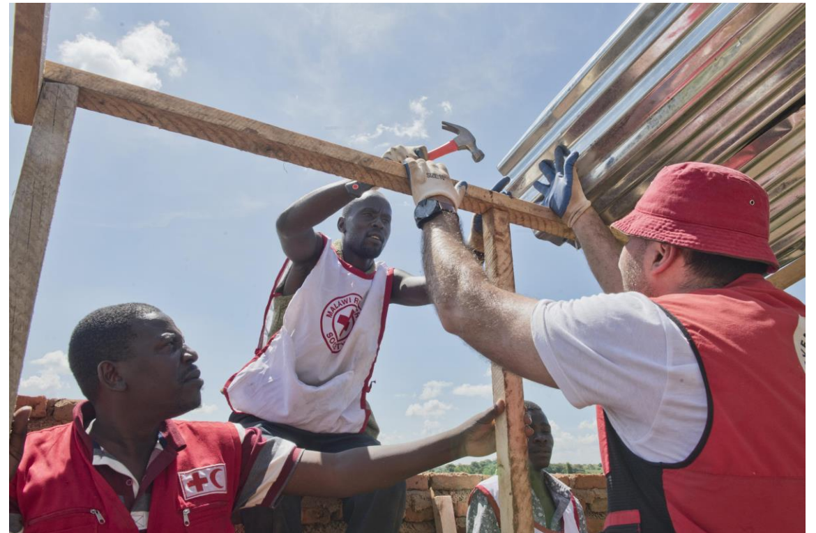
An IFRC delegate and a MRCS volunteer build a latrine in Lilongwe. IFRC
