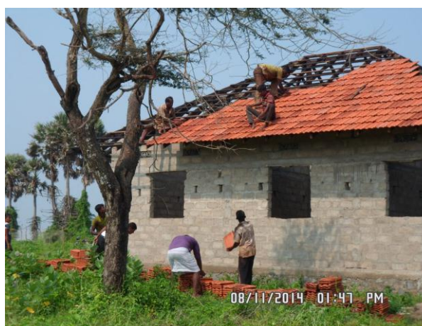
Construction is ongoing in Mr S.Yogendra Pirapus' house in Kokupadayan, Mannar. Photo cred: S. Umakanthan (IFRC)
