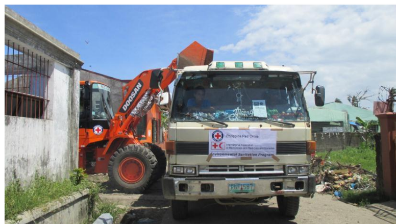
Environmental sanitation and the cleaning of debris in Leyte: Of all the areas hit, Leyte sustained the most damage by Typhoon Haiyan, especially in Tacloban City and coastal areas. A collective 1,946 cubic meters of debris was removed from the community and household areas using payloaders and trucks supported by PRC, IFRC and partner national societies. (Photo: PRC/IFRC)
