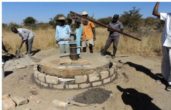
Water point in Mzimuni being rehabilitated. Borehole has not been working for the last 2 years and people were collecting water from a river 3 km away
