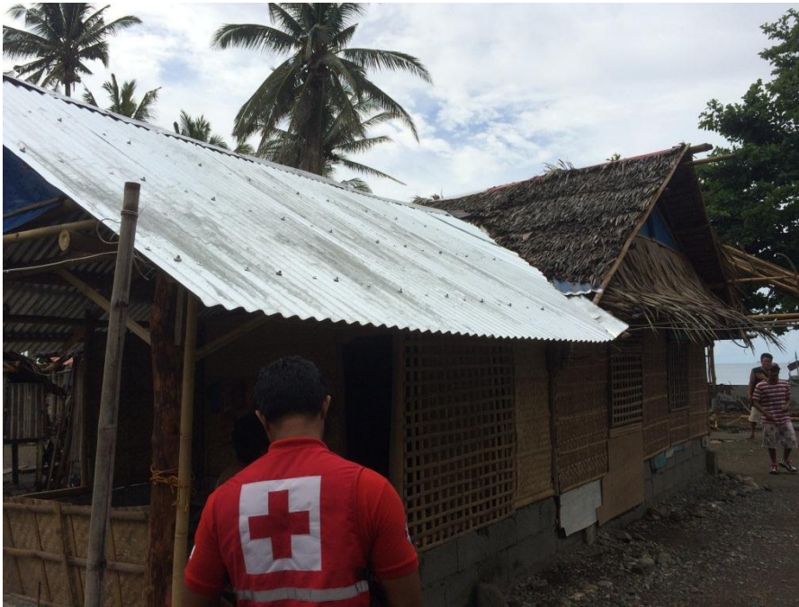
Inspection of the final work on a house which was rebuilt with shelter repair assistance under this operation. PRC volunteers and IFRC technical staff continue conducting such inspections to ascertain how well build back safer techniques have been used. (Photo: Wardell Eastwood/IFRC)
