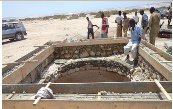
SRCS staff monitoring the rehabilitation work of shallow well in Hafun district. Photo by SRCS
