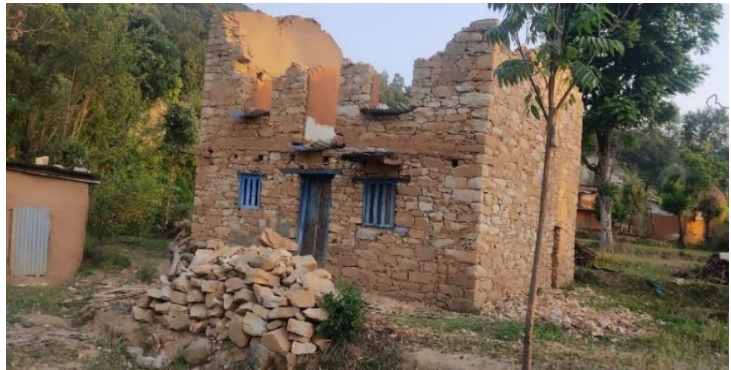
Figure 2: A house damaged by earthquake.
