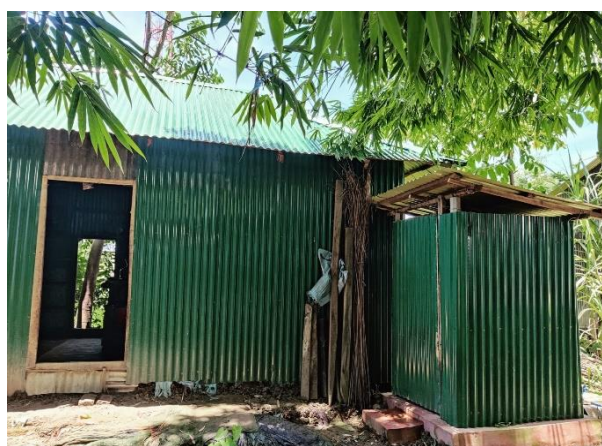
Photograph 1: One of the shelters built with CGI sheets and conditional cash grants under Flood Operation, 2022
