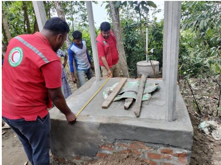
Photograph 3: Shelter and latrine construction process was constantly monitored by the BDRCS NDRT and NDWRT members, Volunteers and other officials
