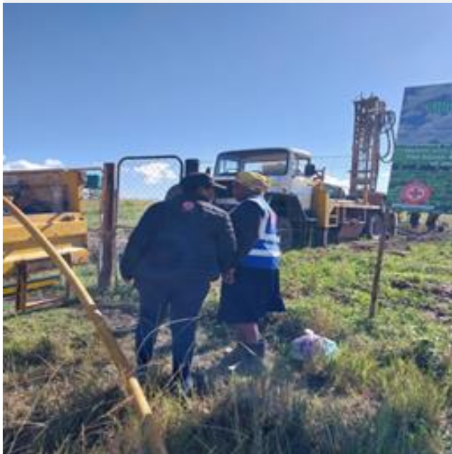
Figure 3: SARCS drilling borehole and installing solar panel pump at Sibusiso Mahlangu Food Garden
