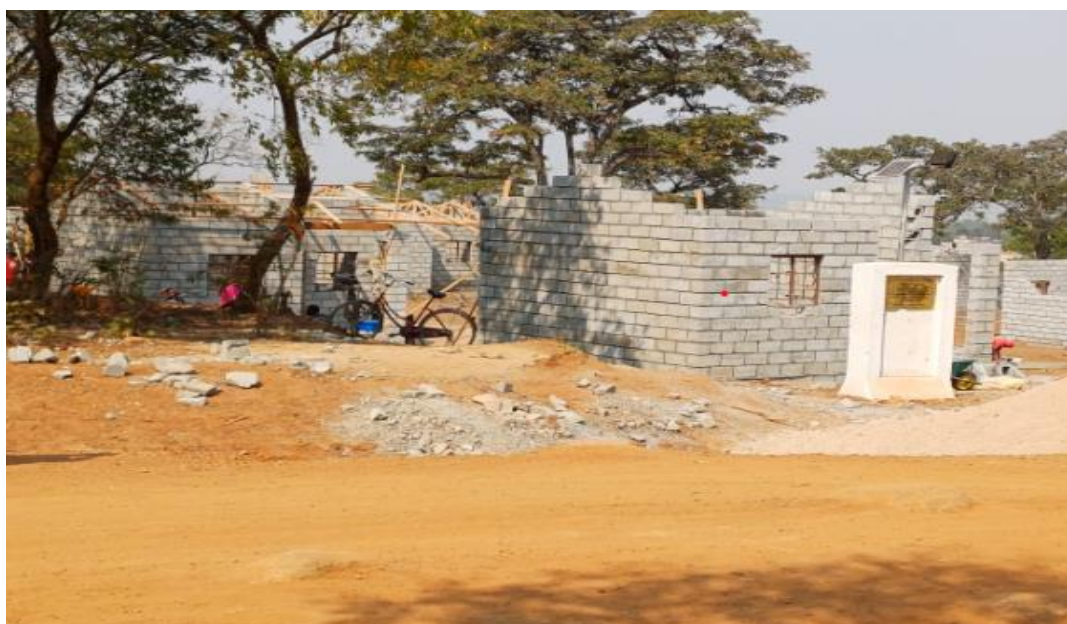
Construction of the 45 houses under emergency Appeal is at the roofing stage at Phweremwe in Phalombe District
