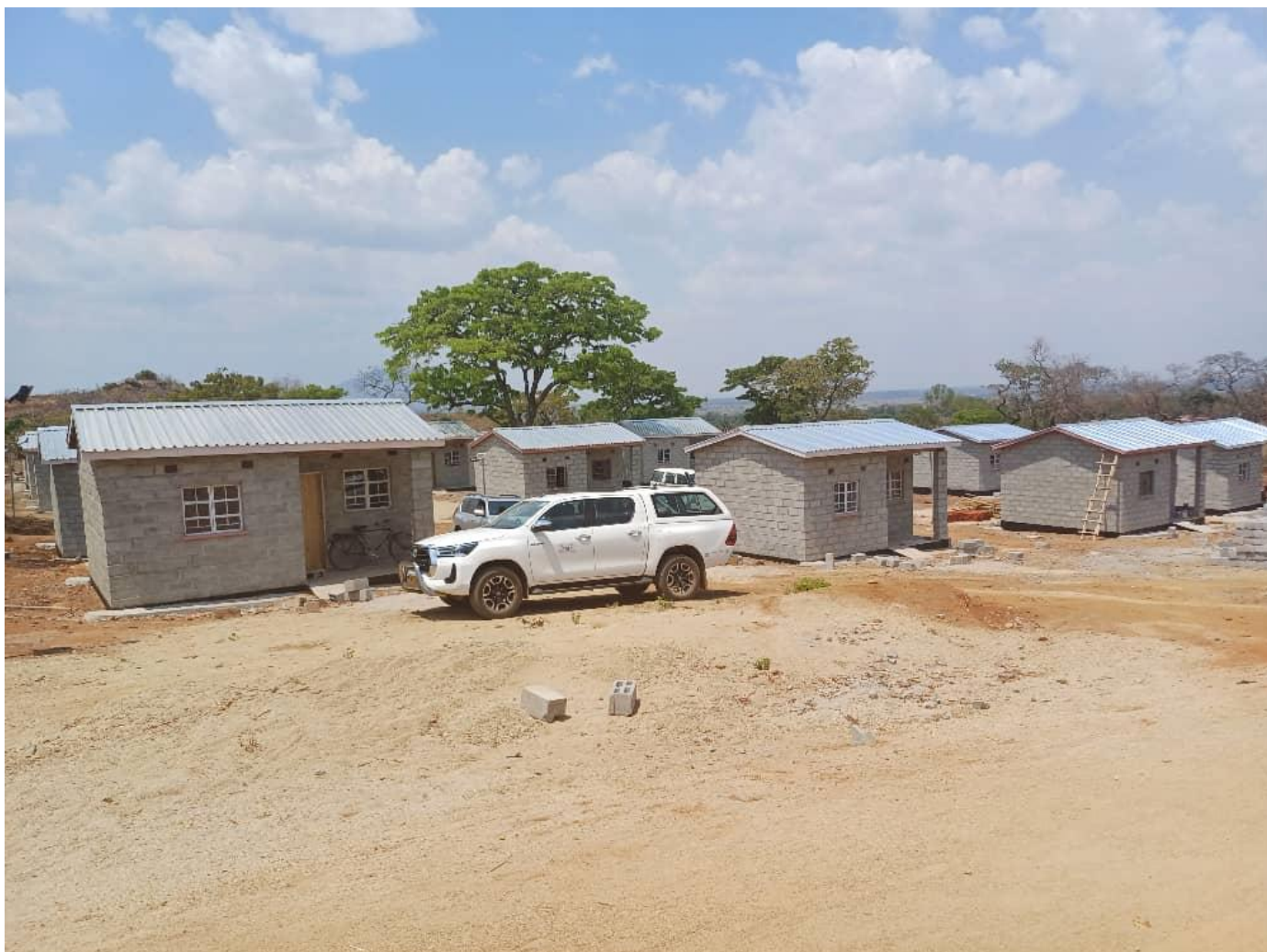
Part of the construction of the houses under Emergency Appeal in Phalombe. A total of 145 houses are to be constructed by December 2023.
