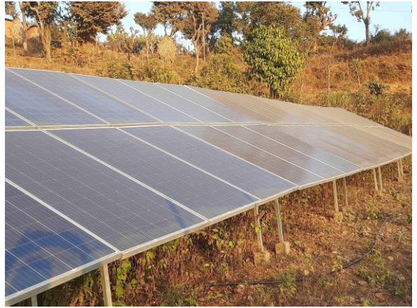
Solar system in Rampur, Ramechhap 5
