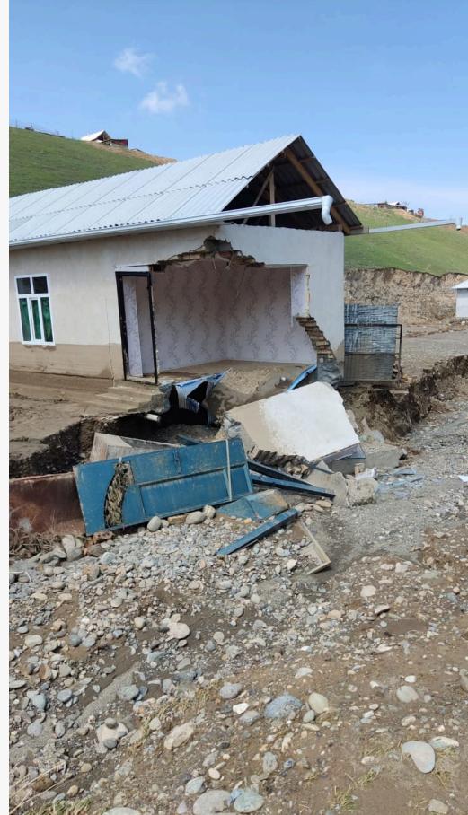
The mudflows have extensively damaged or destroyed houses. Photo credit: RCSK
