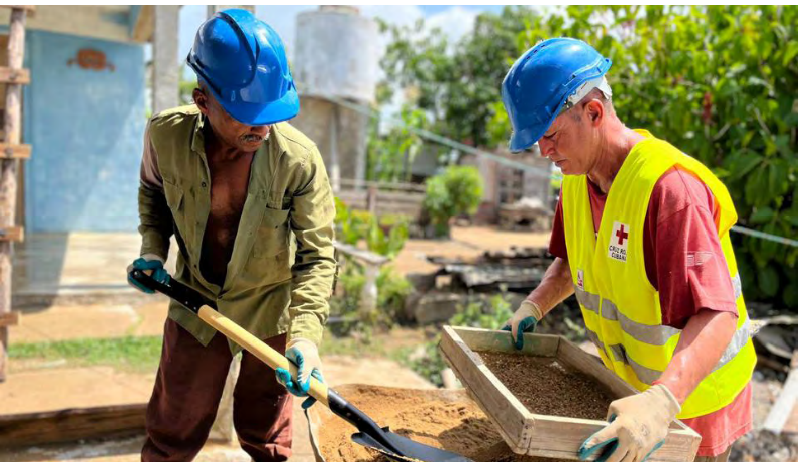
Roof brigades of the Cuban Red Cross in Consolación del Sur assisting communities in rebuilding after Hurricane Ian, 8 March 2024. (Photo: Cuban Red Cross/Susana Arroyo)
