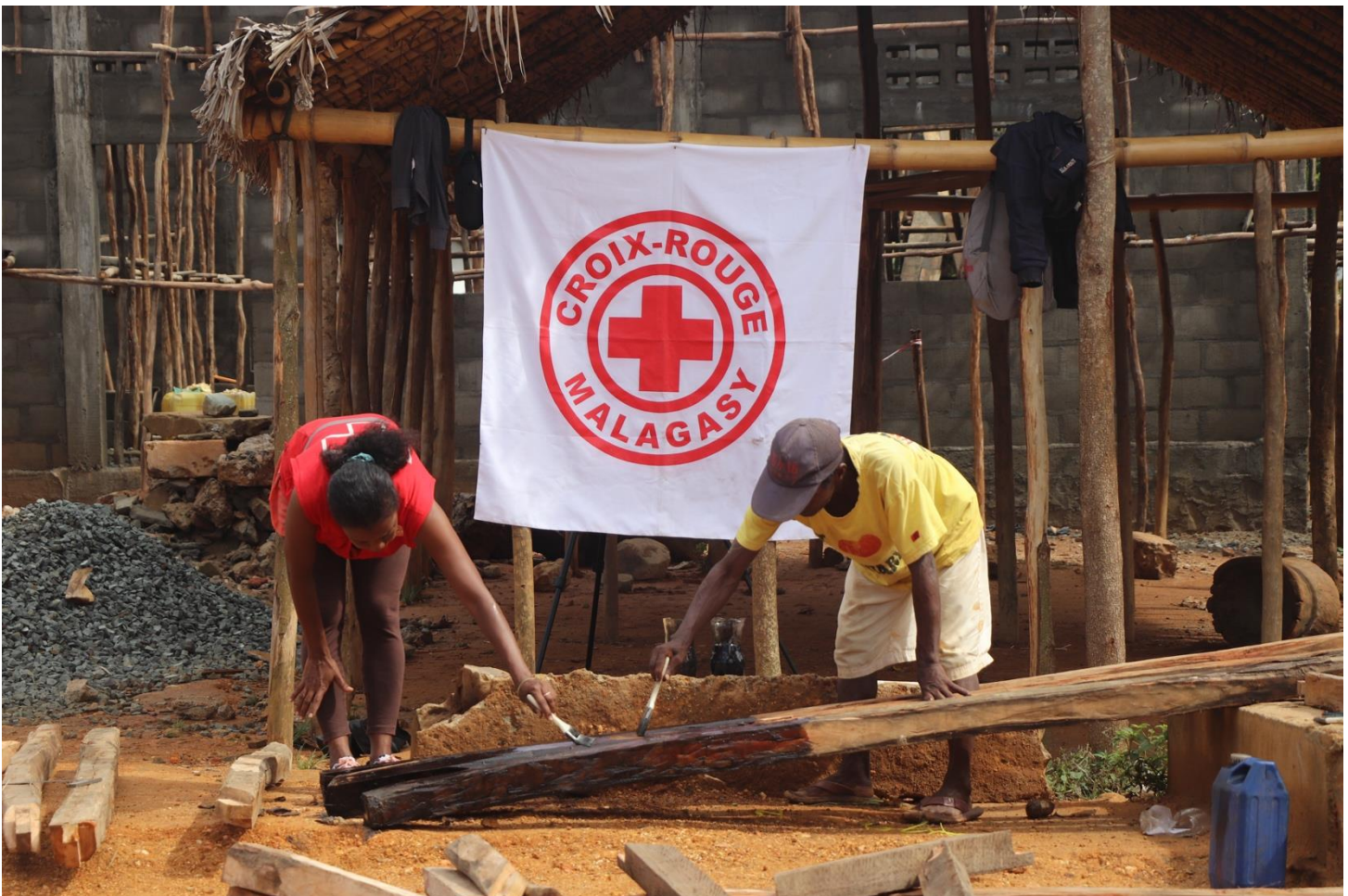
Hut reconstruction in Tsaravary with MRCS paracyclonic norm (Southeast of Madagascar) in partnership with the communities and the volunteers.
