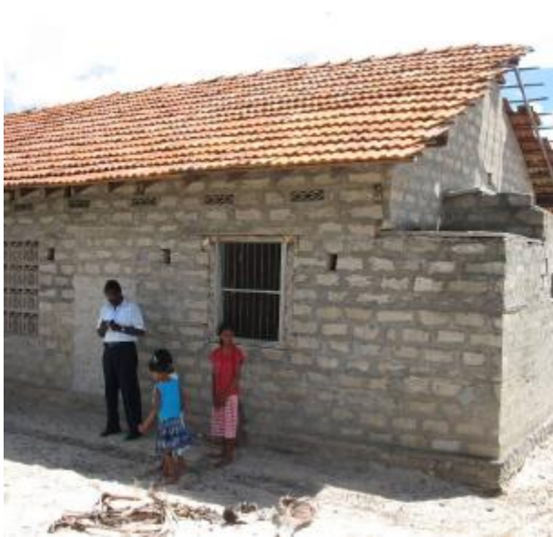
Unfinished house in Jaffna – Kudathanai (without chimney)
