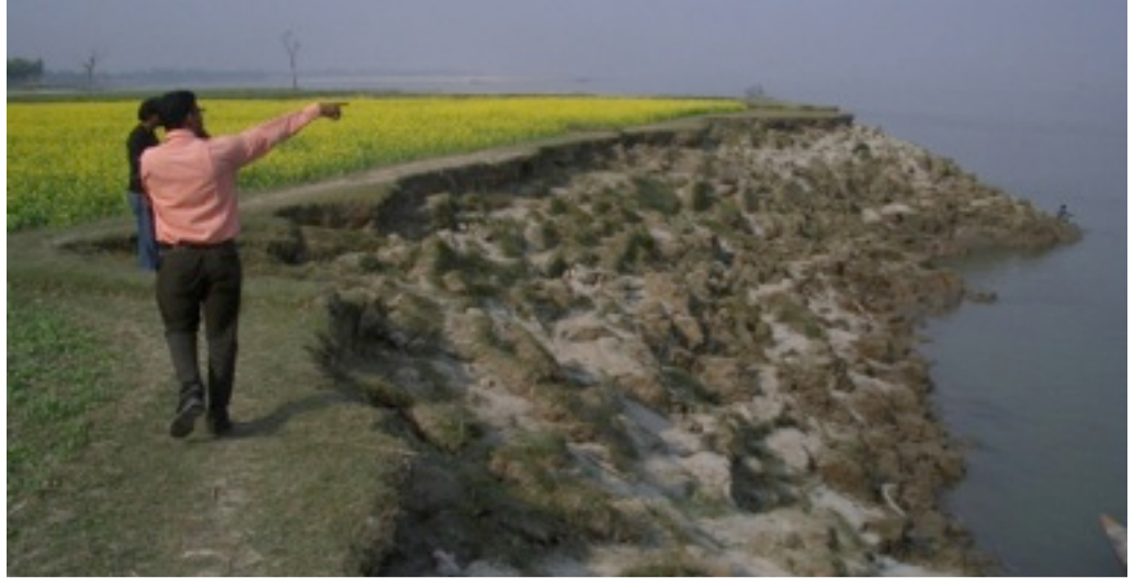
Riverbank erosion diminishes the arable land across most visited communities.
