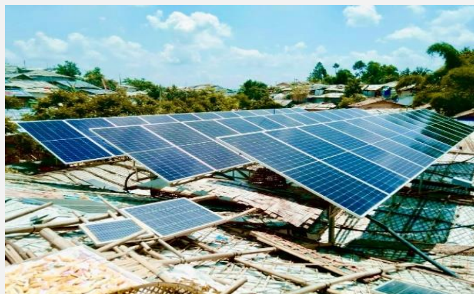
Newly installed Solar System for the last water network in Camp 11 (Photo: IFRC)
